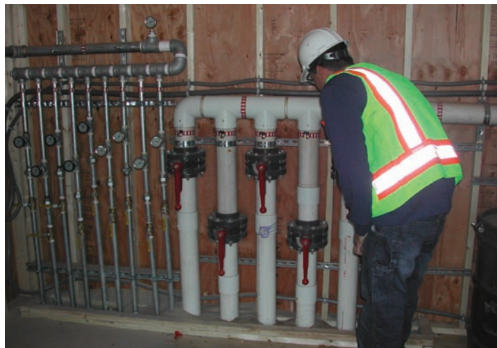
LBG field technician reading vacuum measurements from gauges on the system piping. Steel AS piping is on the left side of the photo.
