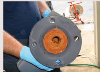
Iron bacteria growth in the groundwater remediation system influent piping
